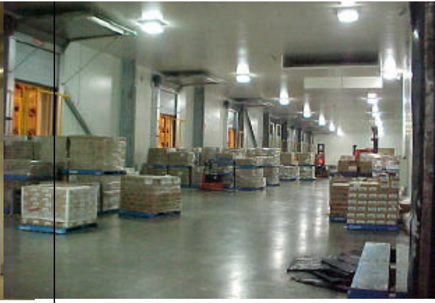
Figure 3 – Loading dock operation, showing high speed insulated doors.
