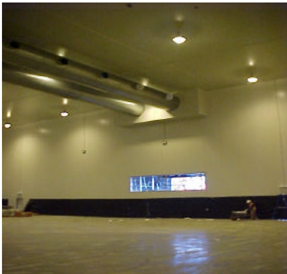
Figure 11 – Room return air aperture and supply air ducting, shown during construction. Racking not yet installed.
